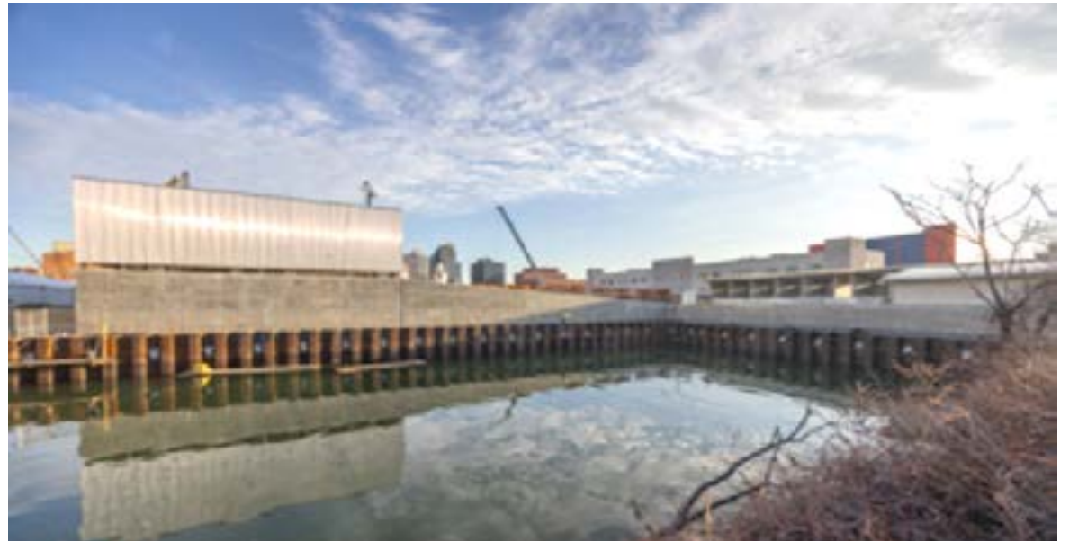
◆ Completed facilities viewed from the Gowanus Canal's 6th Street Turning Basin
