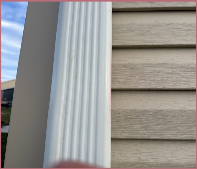
House - Back gutter photo
