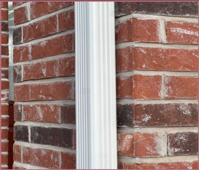
House - Front gutter photo
