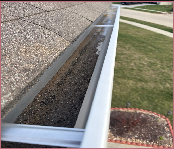
House - Front gutter photo
