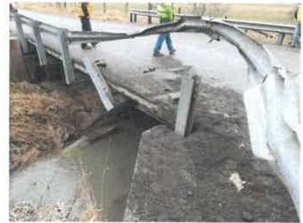
Guardrail damage from tractor trailer on Chapel Rd., CR 63. Repaired by County forces and re-opened to traffic in under 4 hours.
