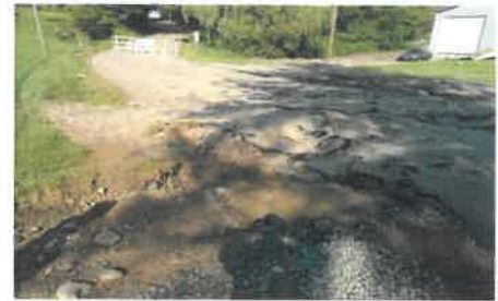
Road damage from pond dam failure on Brass Rd., CR 36. Repaired by County forces and re-opened to traffic in one day.
