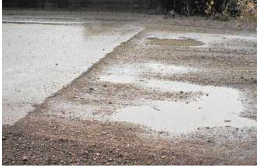
The grader must fill potholes and depressions formed near the bridge approach.
