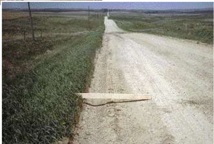
Secondary ditch over six inches deep.
