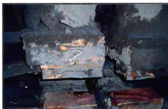
Figure 13 – Poorly maintained and worn copper jaws
